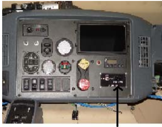
I.R. Control Panel
